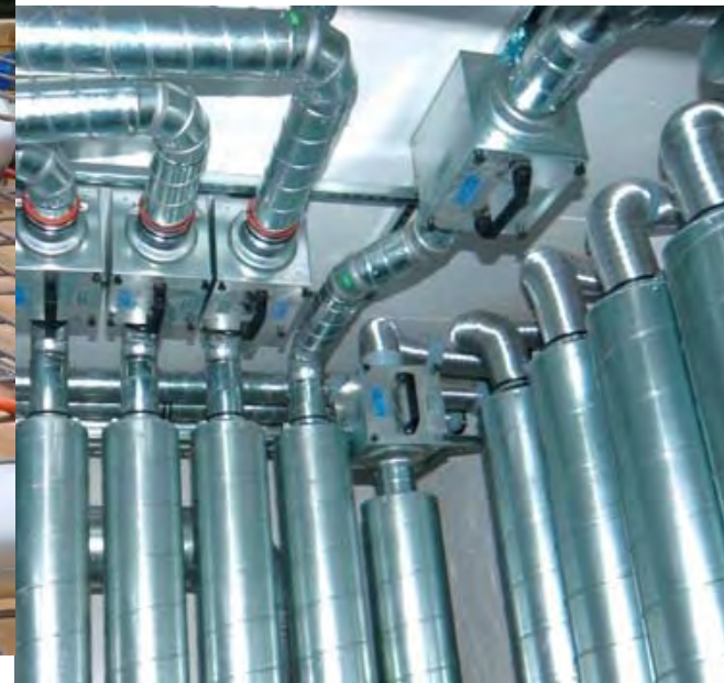
In the technical room
