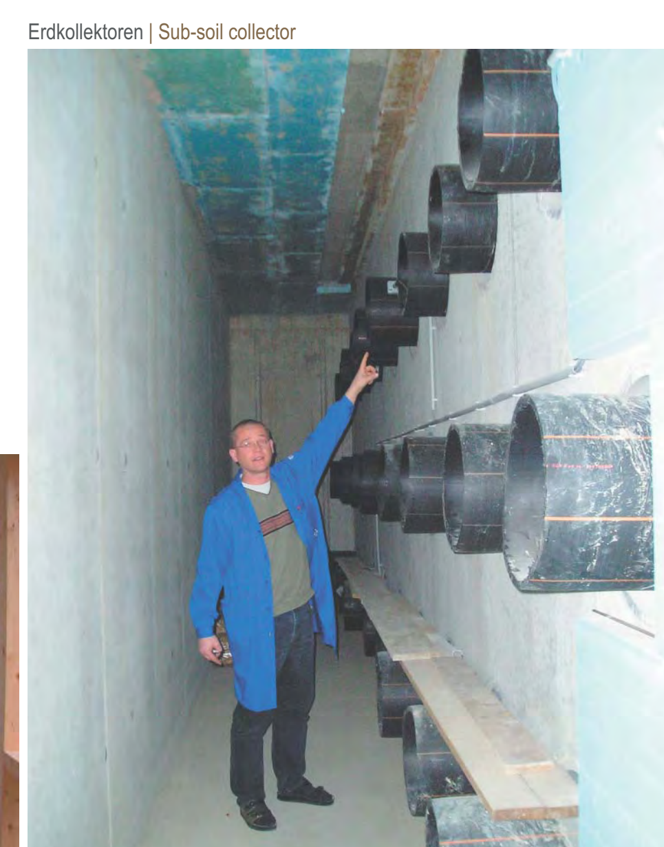
Erdkollektoren | Sub-soil collector
