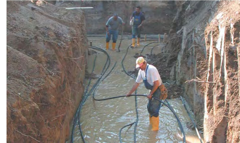
Sole-Erdkollektor | Brine sub-soil collector
