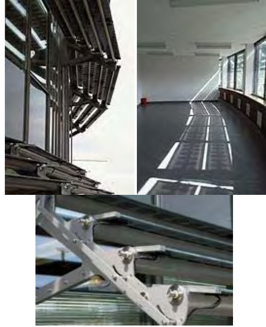
Abbildung 24: Colt Shadovoltaik am SBL Offices Linz © Colt
